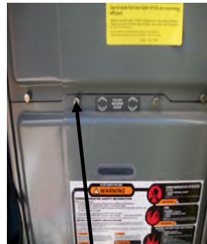
Access Panel (Town Homes)
